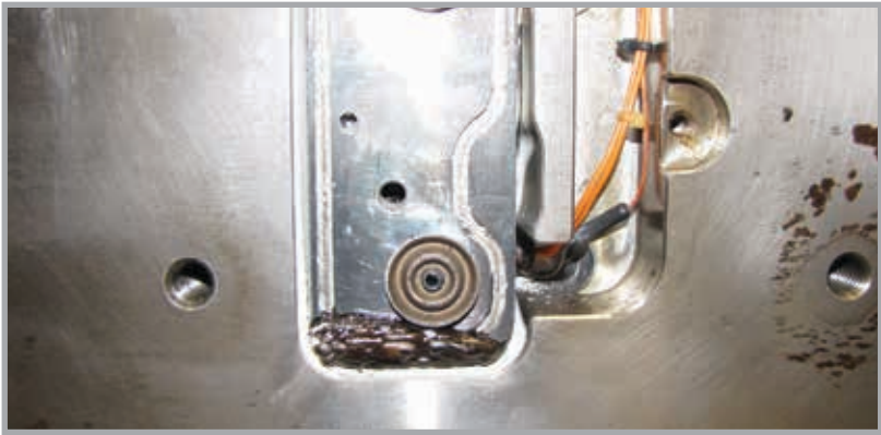
Actual Leak Detected with Alarm
